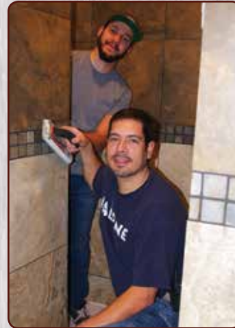
Ben and Dane put finishing touches on the most recent Cedar Restroom remodel
